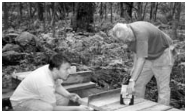
Jeff Rutter with his father, Bruce, work on one of the new bridges crossing wet areas.
